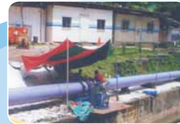
Purple ProFuse for NEWater, Singapore First large diameter polyethylene installation in Singapore as traditional metallic material proved unsuitable for above ground waste water use
