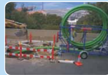
Green ProFuse for Lyonnaise des Eaux, Gibraltar Sea water mains replacement using sliplining and pipe bursting techniques
