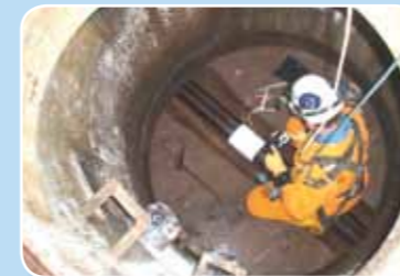
Black ProFuse with a brown stripe for Magnox North Sites, UK Effluent pipe refurbishment at nuclear power station using sliplining technique
