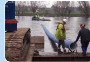
Dark blue ProFuse for Dee Valley Water, UK Sliplining project to replace an existing plate riveted water main beneath the river bed
