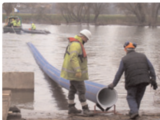
ProFuse pipe being floated into position for a sliplining project in the Dee Valley (UK). The pipe was laid into an existing plate riveted water main beneath the river bed
